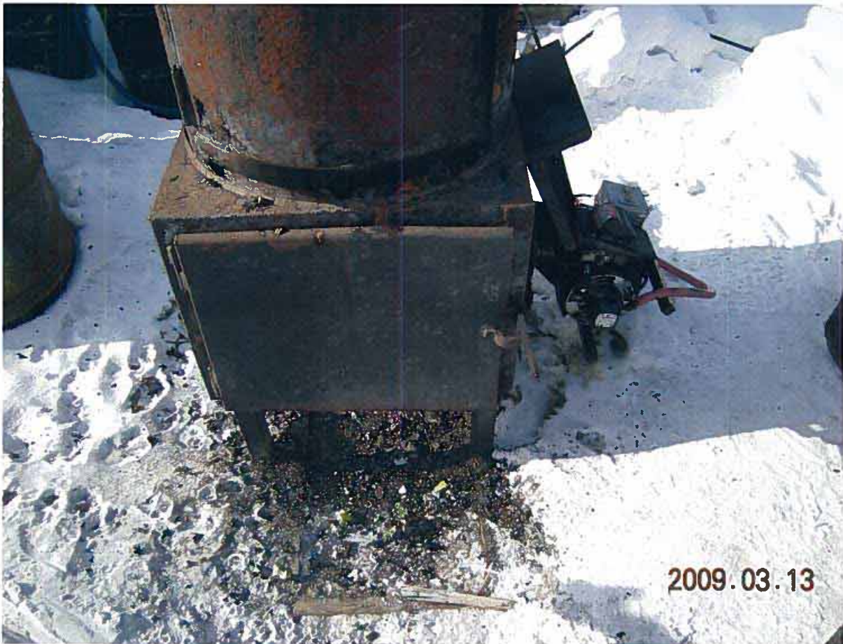
MV2007C0039 - Avalon Ventures Ltd. Small fuel leak to address on the incinerator and a "drip defender" must be placed at this location.
